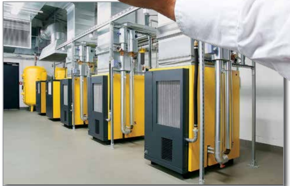
Air-cooled, fluid-injected screw compressors with internal heat exchangers and controls to tap into the thermal energy of the cooling fluid. The additional ducting removes the hot air that was not rejected by the hot water recovery system.
